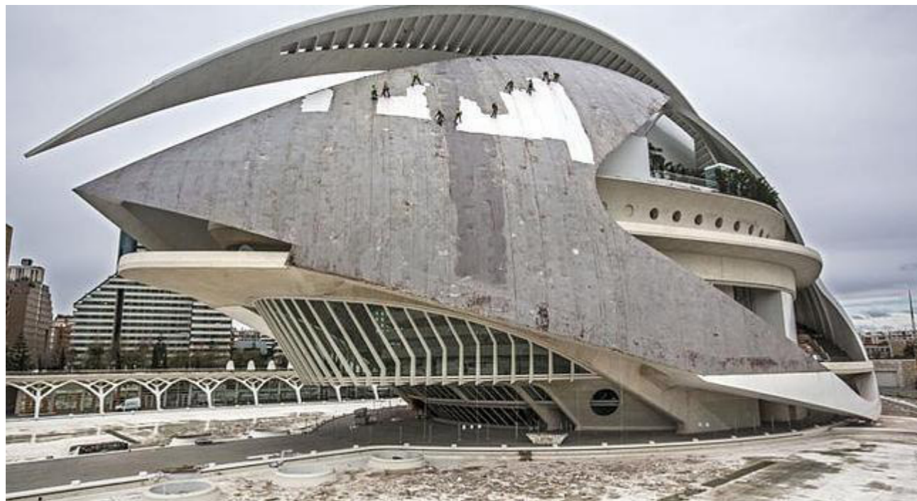
Palau de les Arts (City of Arts and Sciences) Problems on the coatings
